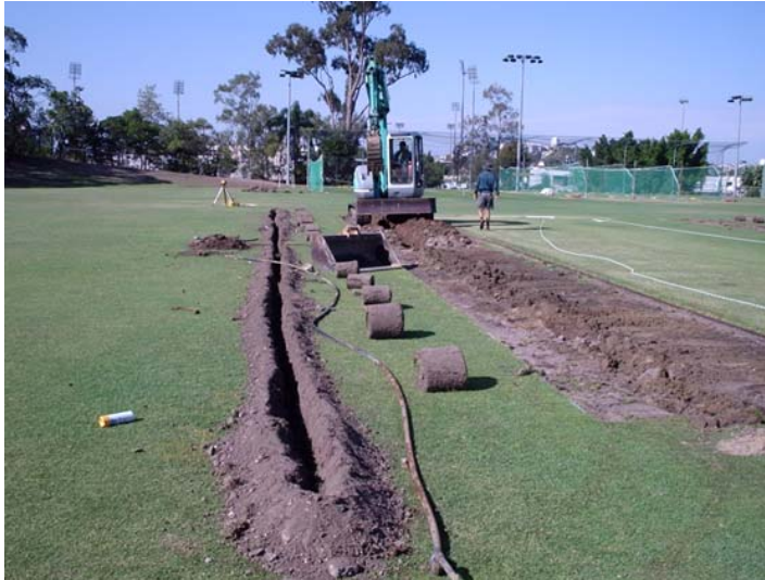
Figure 17: - Irrigation line 3m from Wicket Block
